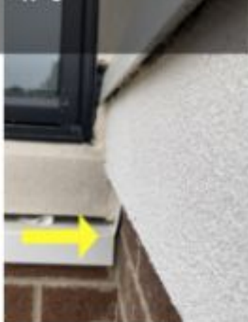
Capping not secured on to bricks
